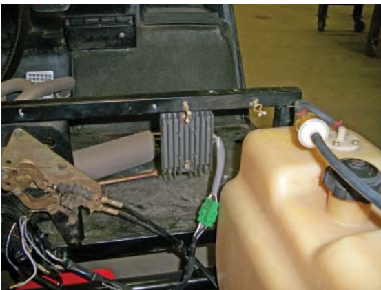
Igniter Mounting Area
